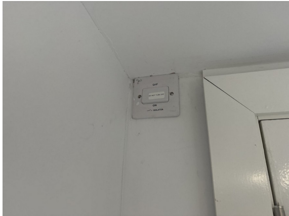
R5-25 | En-suite extractor-fan isolator switch Photographed 21 August 2026 at 15:37
