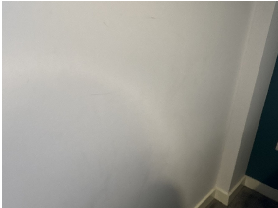
R5-06 | Wall corner - condition detail Photographed 21 August 2026 at 15:34
