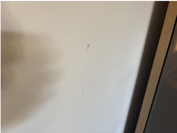
R5-04 | Wall finish - minor mark detail Photographed 21 August 2026 at 15:34
