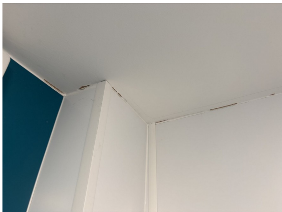
ES-13 | Separate area of lifted sealant and paintwork at wall/ceiling corner Photographed 21 August 2026 at 15:43
