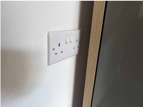
R5-28 | Double electrical socket - condition detail Photographed 21 August 2026 at 15:44
