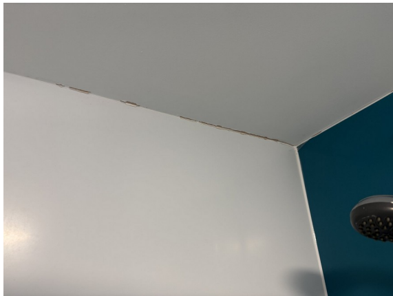
ES-11 | Sealant and paintwork at ceiling corner Photographed 21 August 2026 at 15:43
