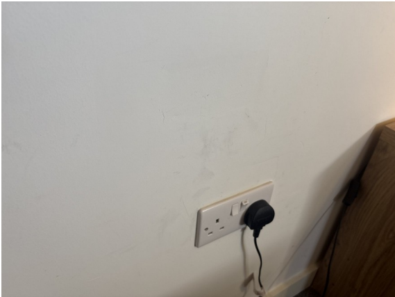
R5-02 | Wall and electrical socket - condition detail Photographed 21 August 2026 at 15:33
