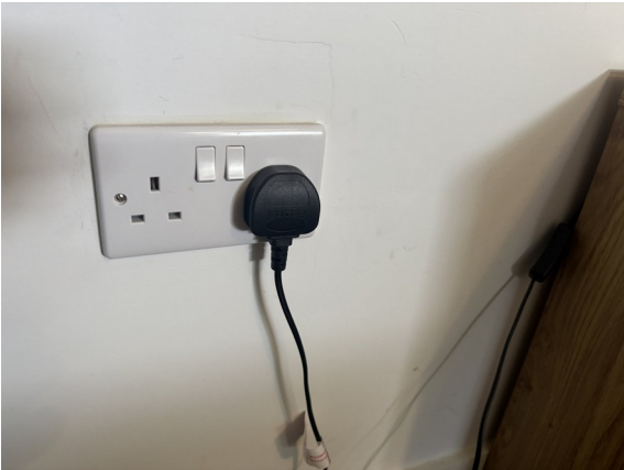
R5-29 | Double electrical socket and adjacent wall mark Photographed 21 August 2026 at 15:44
