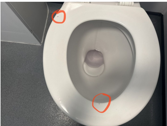
ES-14 | Toilet seat - paint-chip condition details Photographed 21 August 2026 at 16:11
