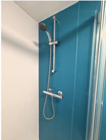
ES-09 | Shower controls, hose and wall finish Photographed 21 August 2026 at 15:41
