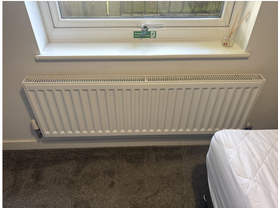
R5-21 | Radiator beneath window Photographed 21 August 2026 at 15:36
