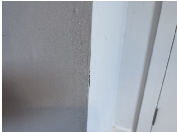
R5-05 | Door and frame - condition detail Photographed 21 August 2026 at 15:34
