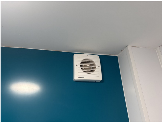
ES-12 | Extractor fan Photographed 21 August 2026 at 15:43
