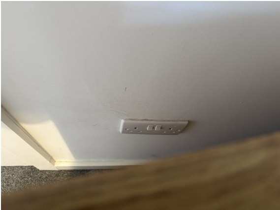
R5-26 | Electrical socket - condition detail Photographed 21 August 2026 at 15:44
